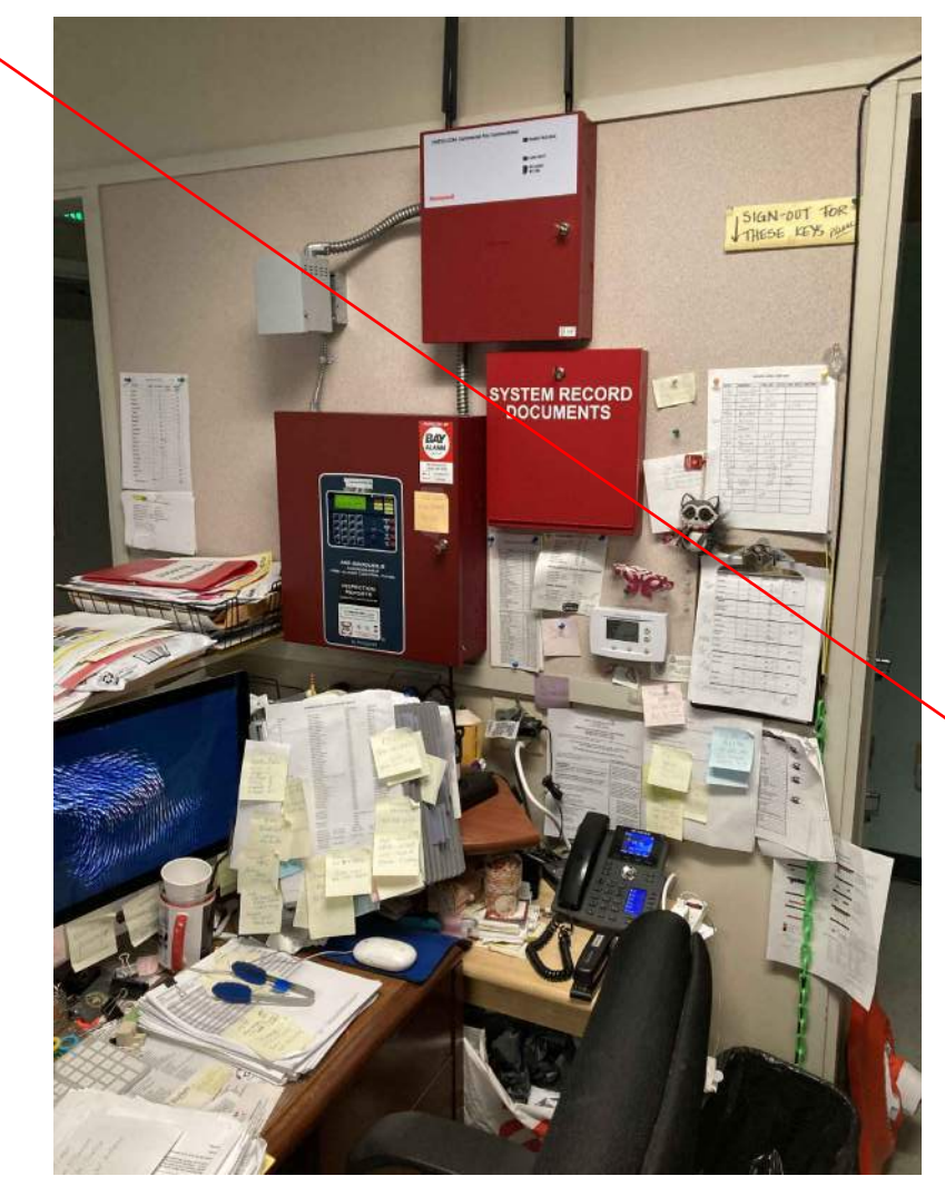
(E) FIRE ALARM PANEL
